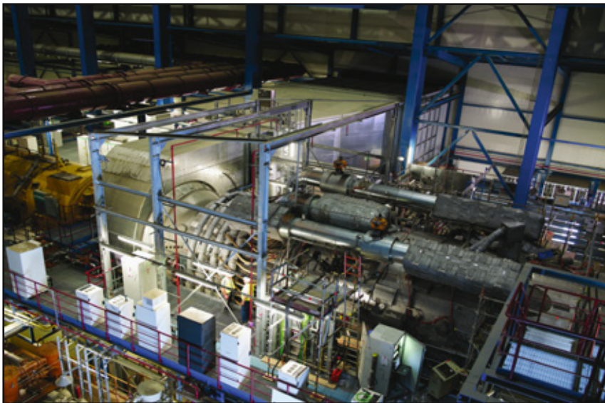
Shown here is the SGT5-8000H gas turbine installed at the Irsching 4 plant. The Irsching test center is property of Siemens and will remain so until the end of the combined-cycle test, when the whole plant will be handed over to E.ON, which will run it as a regular power generation section of the Irsching power plant.
